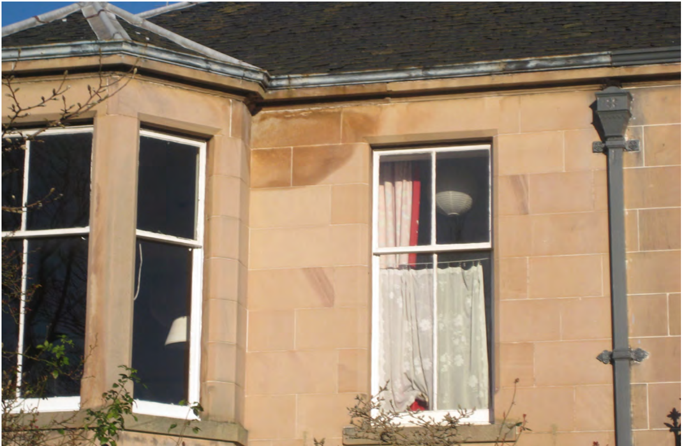
Figure 2: Damp penetration (image © Historic Environment Scotland)
