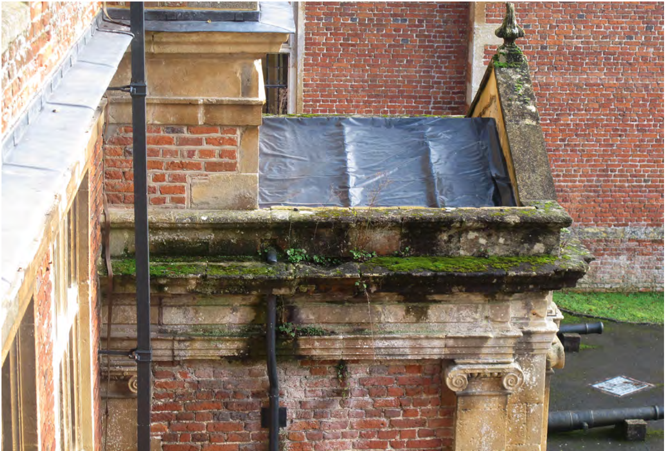
Figure 7: Poor maintenance (image © Historic England)
