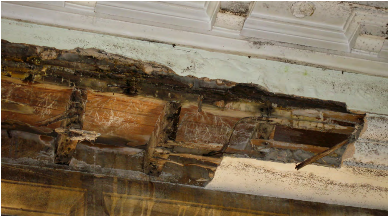
Figure 8: Collapsed plaster due to water penetration via lead parapet gutter (image © Historic England)
