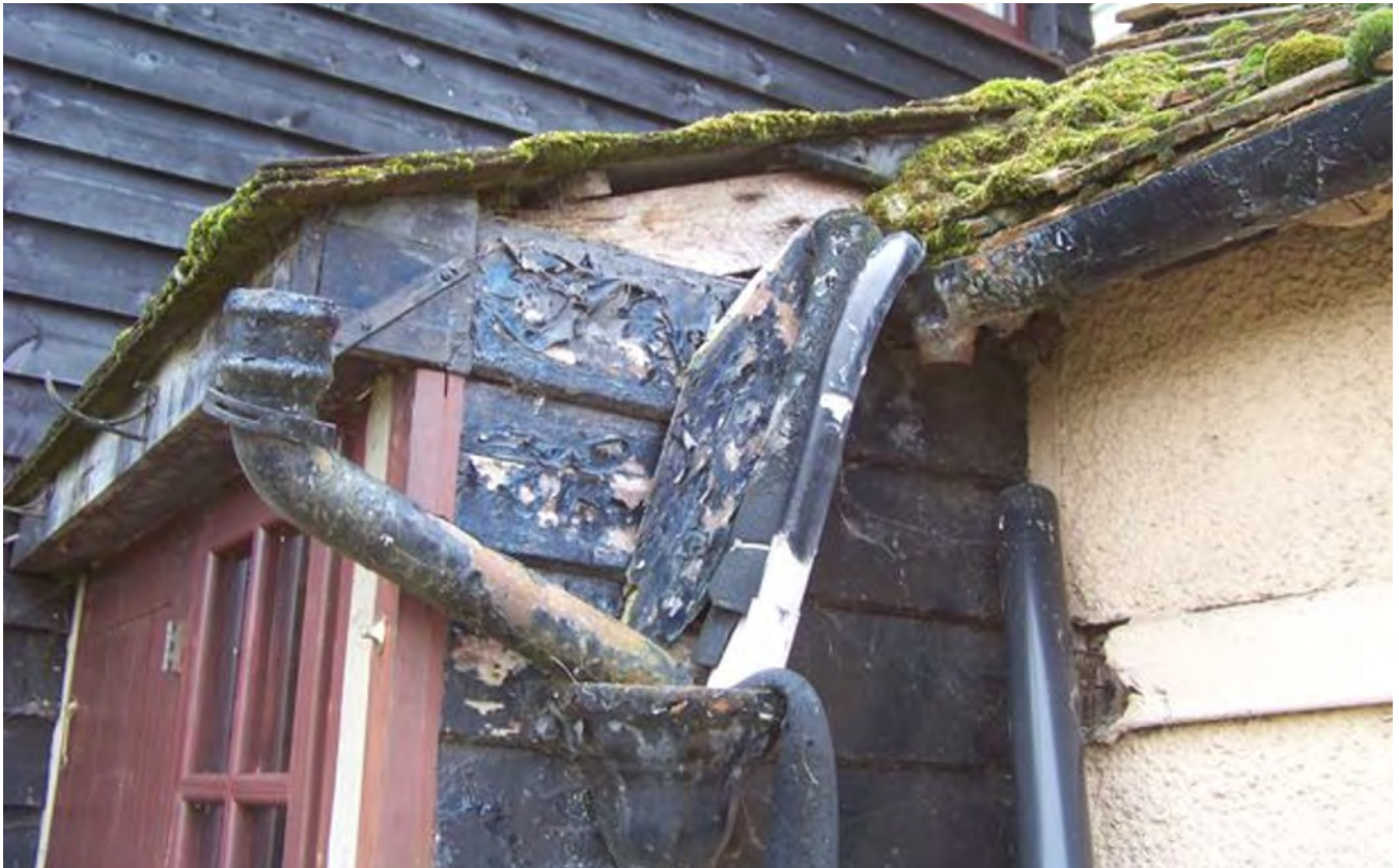
Figure 5: Defective rainwater gutters and downpipes (image © PCA)
