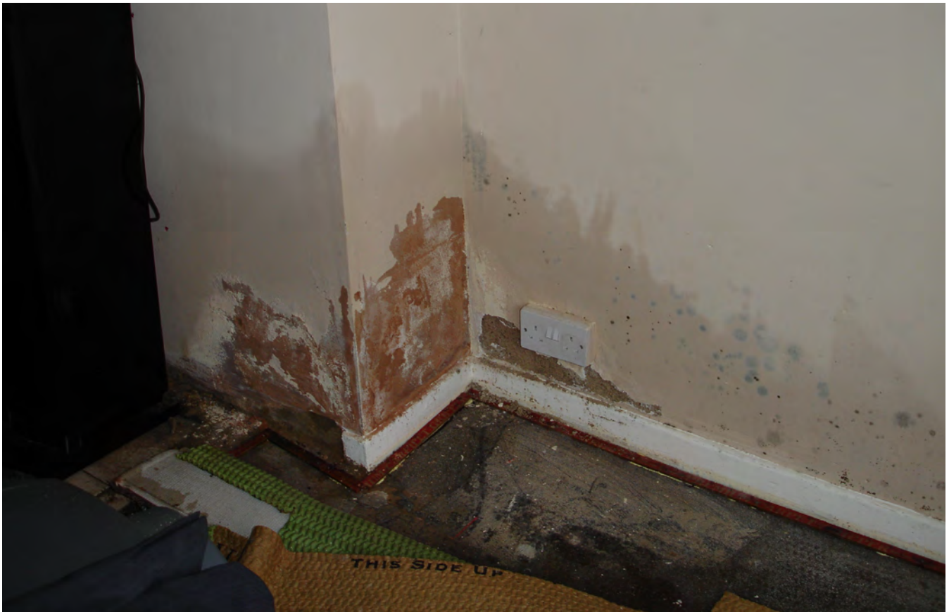
Figure 4: Elevated moisture in a wall (image © PCA)
