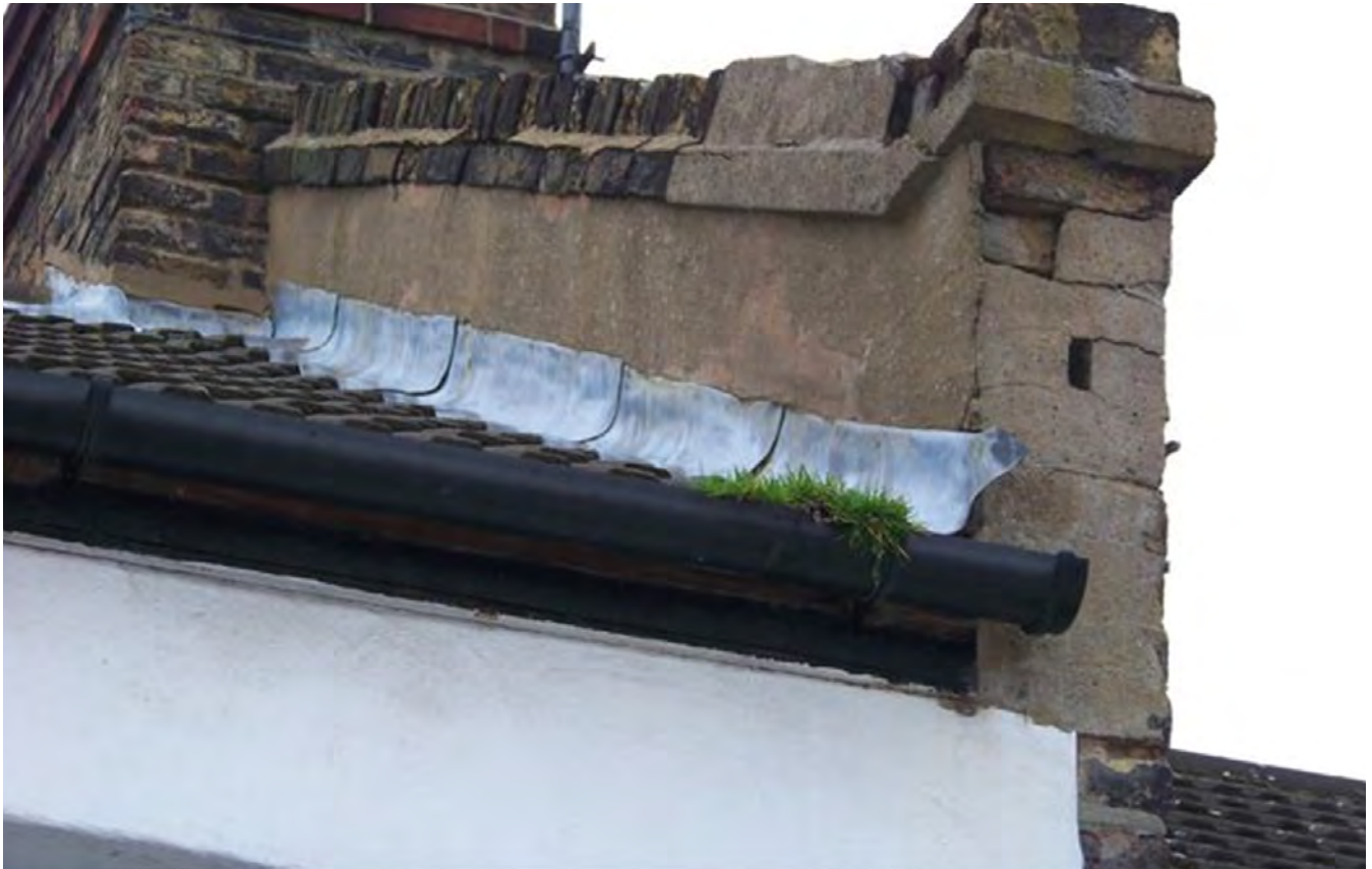
Figure 1: Parapet wall in poor condition (image © PCA)
