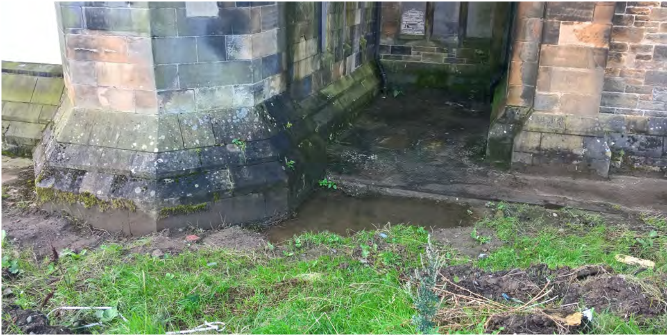
Figure 3: Defective rainwater disposal (image © Historic Environment Scotland)
