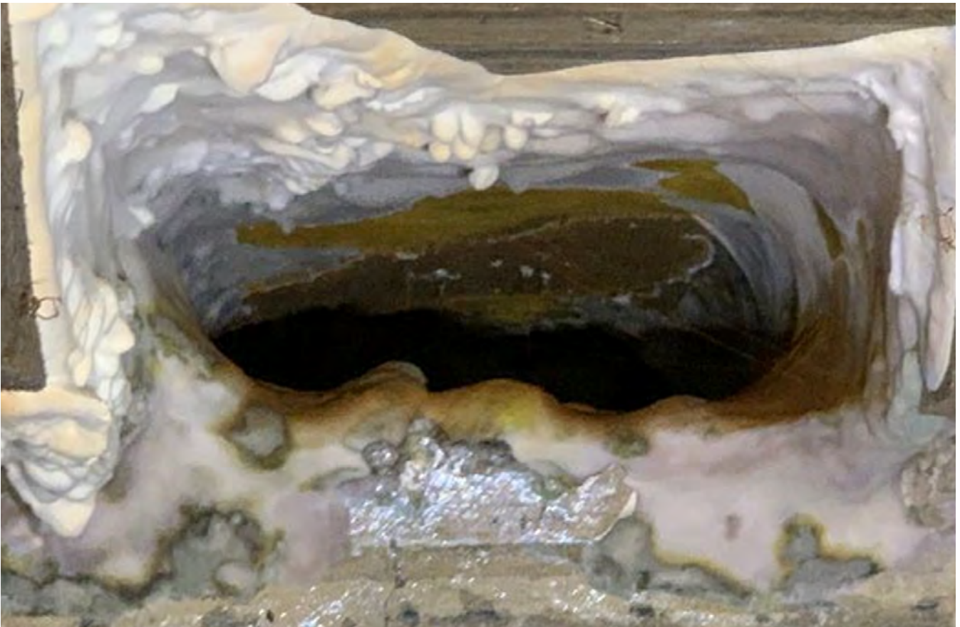
Figure 6: Dry rot under a suspended timber floor (image © RICS)
