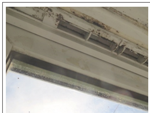
The picture above shows a trickle vent which was stuck to the window frame but without sufficient opening.
