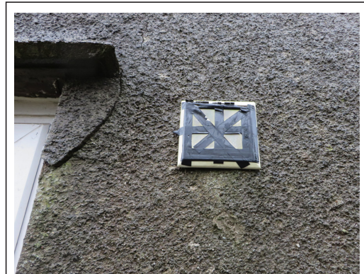
An example of an intermittent fan which had been covered by the occupant. In many instances the alterations may not be so obvious.
