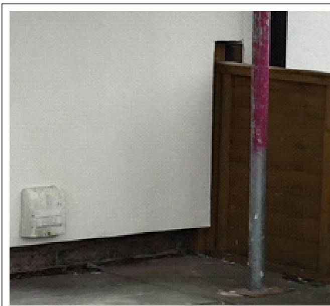
External wall insulation applied to a solid wall structure. Note the breaks in continuity of the insulation firstly where the fence intersects the insulation and secondly at the base of the wall, where the insulation has not been continued to ground level.
