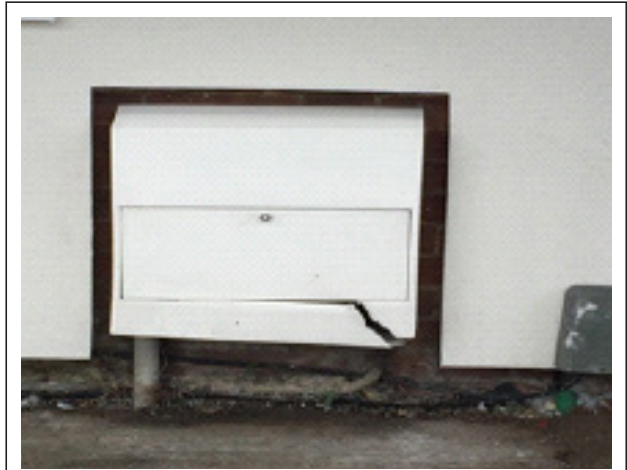
Another example of discontinuous insulation which will result in temperature differentials in the structure and may result in condensation and mould growth problems.
